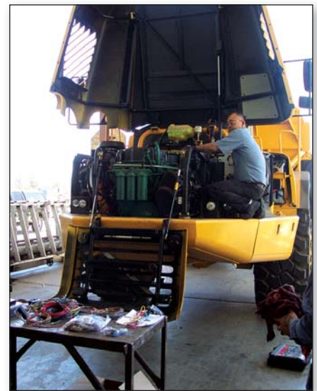
Ted Hada, an employee of West-Mark, Ceres, Calif., installing a TAS system on a new Volvo A-40 Articulating Dump Truck for ASRC.
